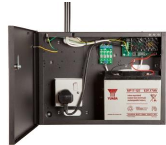
Optional black XLB box with the door & sides replaced & equipment installed
