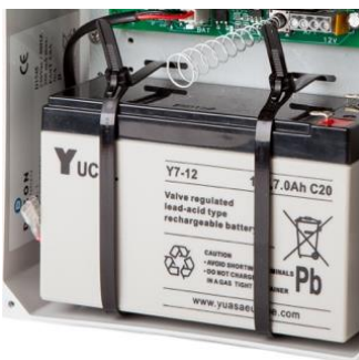
Battery restraining ties
