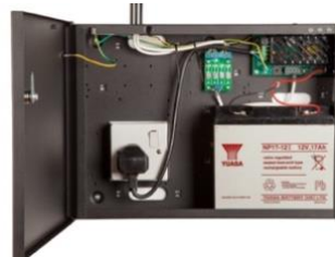
Stage 3 - a 17Ah battery & the lid have been fitted
