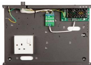
Stage 2 - a 4-way output splitter has been added using the pre-drilled holes
